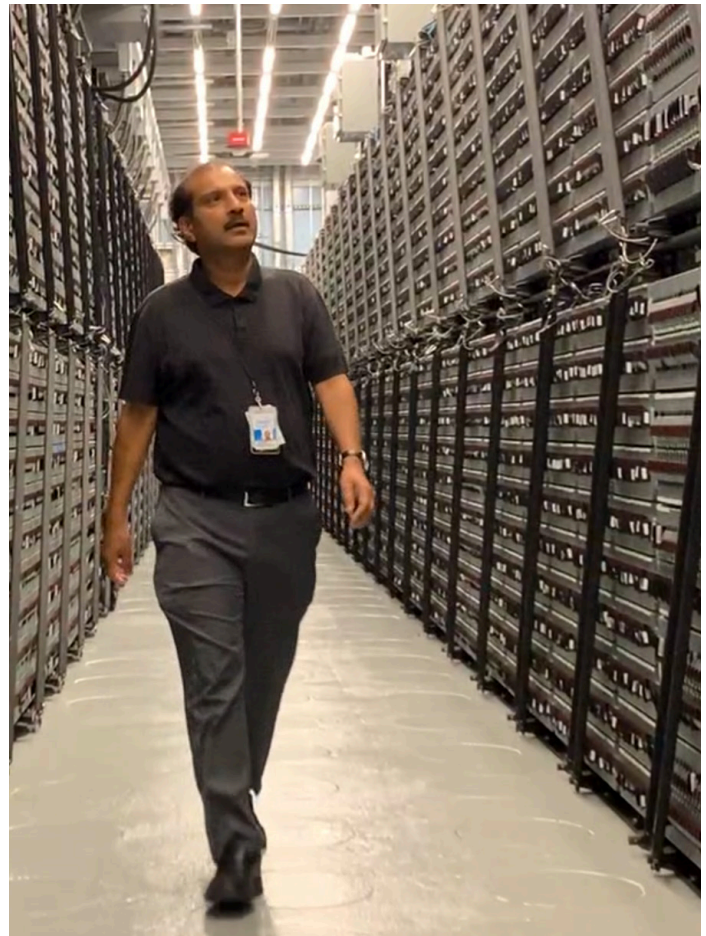
Intel Data Center: 31 MW in 30K SQ FT: 1.06 PUE
